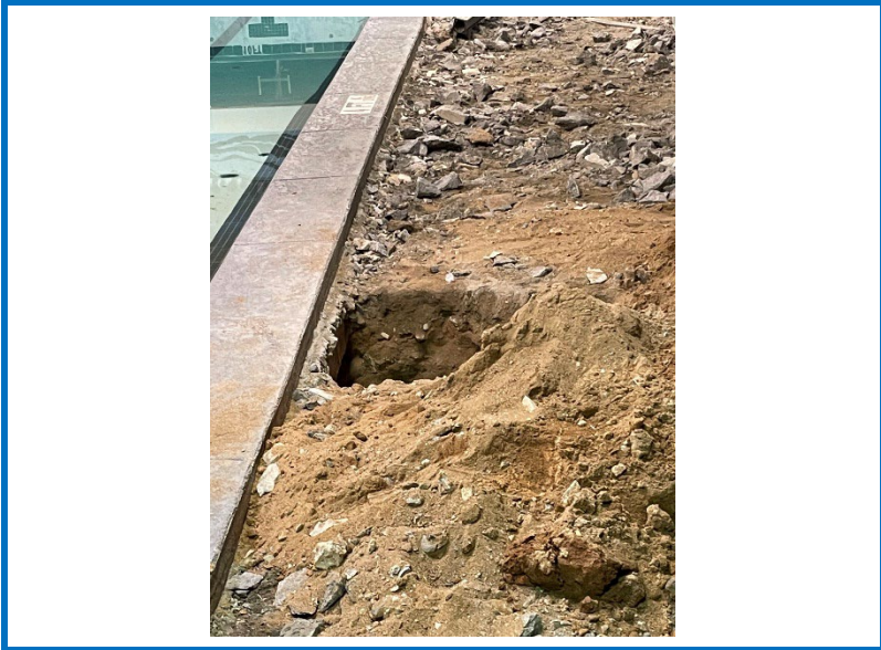
Photo 3: Excavation at inlet pipe leak. View from N. 2/2023
