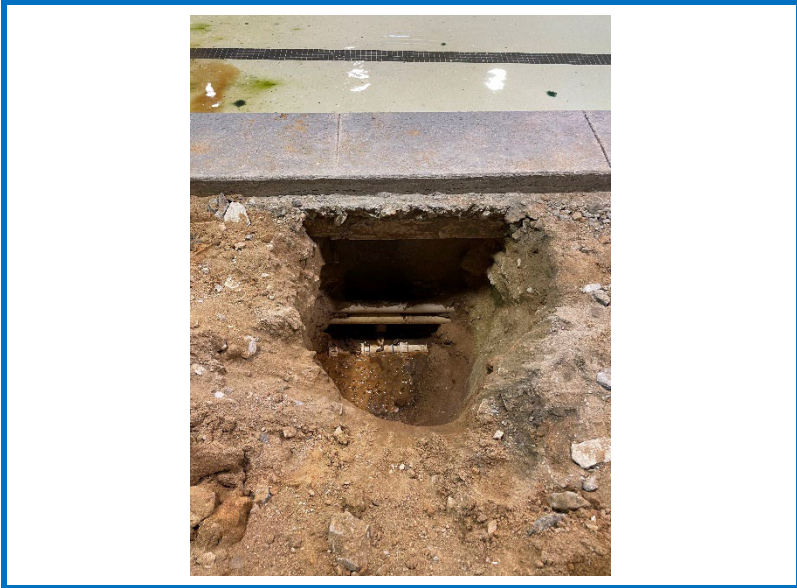
Photo 4: Excavation at inlet pipe leak. View from W. 2/2023
