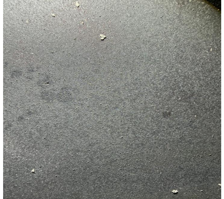
Substrate condition beneath existing coating. Picture #2
