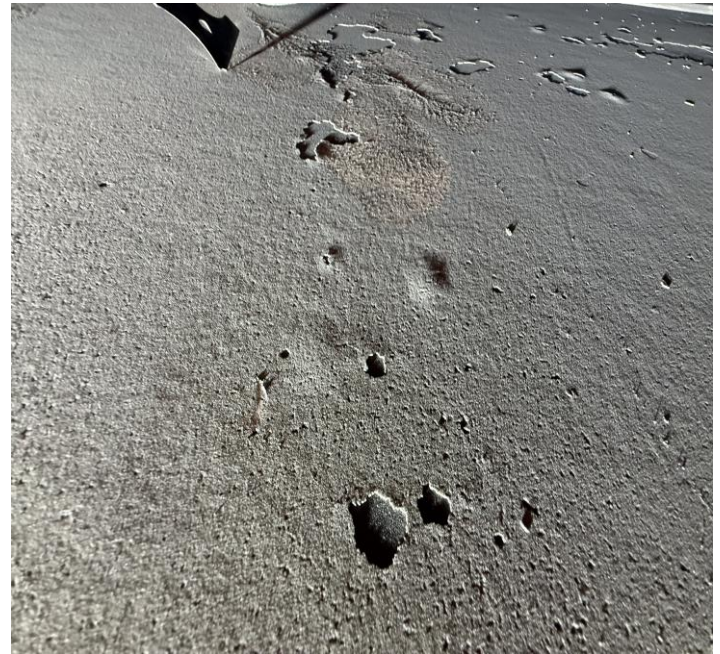
Visible blisters that remained intact after a sweeping blast. Picture #1
