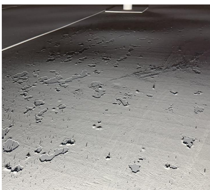
Widespread disbondment observed in large areas of the floor. All edges lifting with poor adhesion. Picture #4
