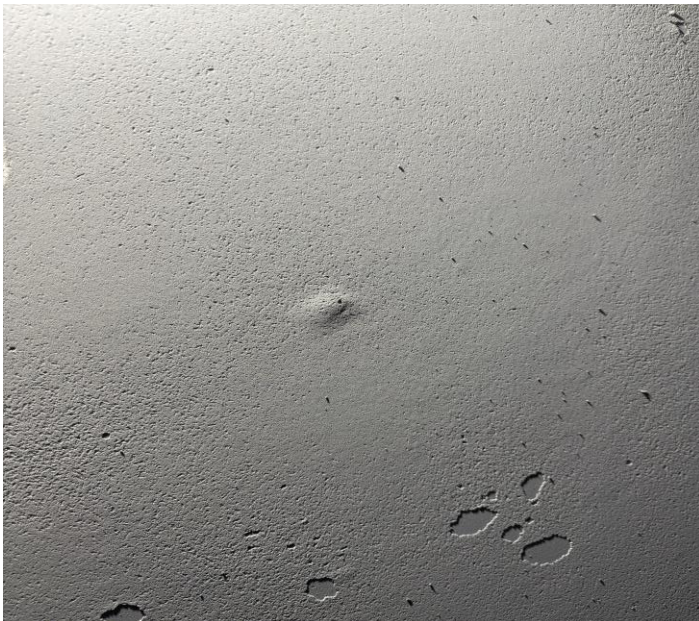
Visible blisters that remained intact after a sweeping blast. Picture #2
