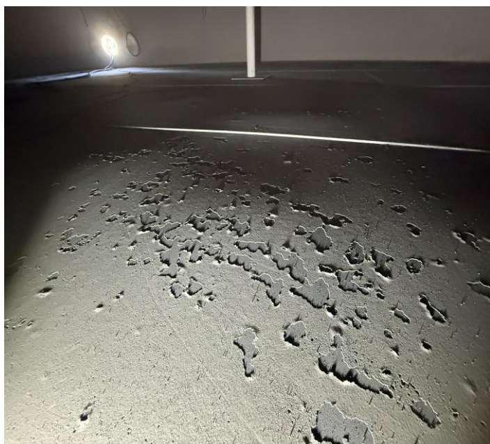
Widespread disbondment observed in large areas of the floor. All edges lifting with poor adhesion. Picture #2
