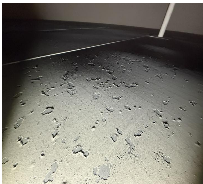
Widespread disbondment observed in large areas of the floor. All edges lifting with poor adhesion. Picture #3
