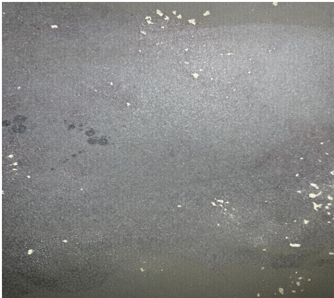
Substrate condition beneath existing coating. Picture #1
