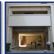
Vertical Lift Flood Barrier
