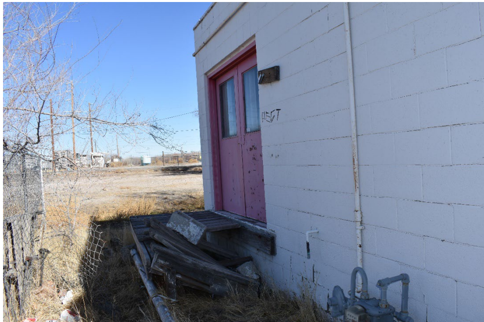
VIEW OF A DILAPIDATED STAIRWAY LOCATED ON THE WEST SIDE OF THE SUBJECT BUILDING
