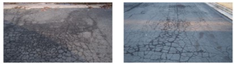
Pavement Condition 11 - 40 (Very Poor/Serious)
