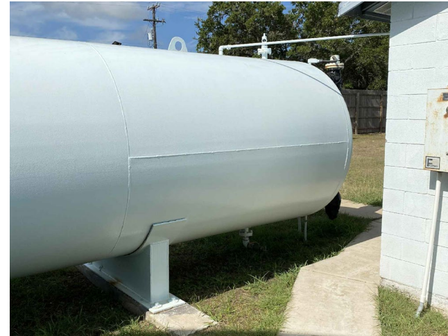
Existing 5,000 gallon hydropneumatic tank at Plant #2
