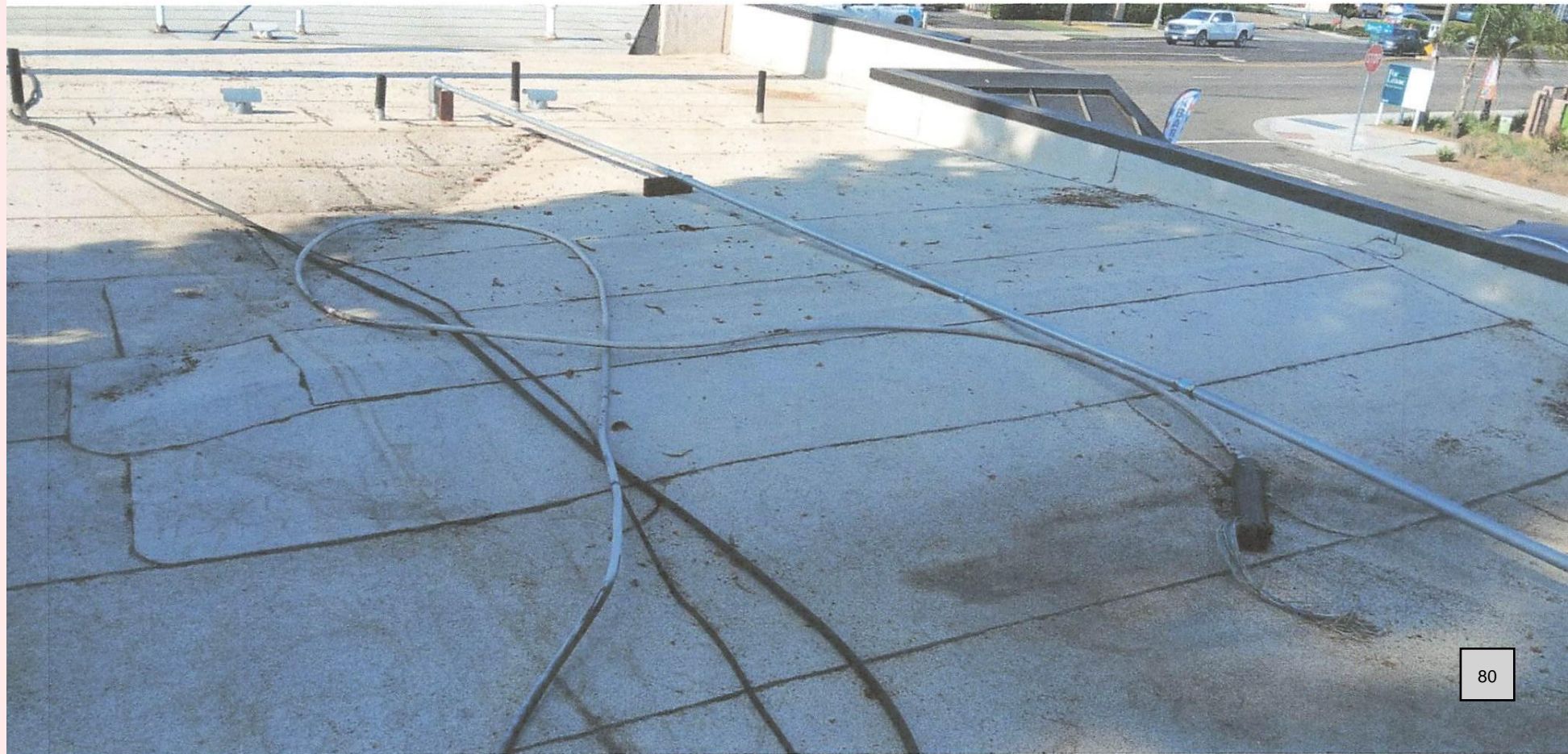
Roof Cleared of Tree Limbs
