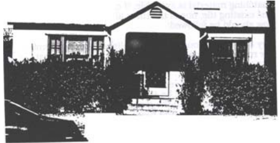
Composition roof needs repair.
