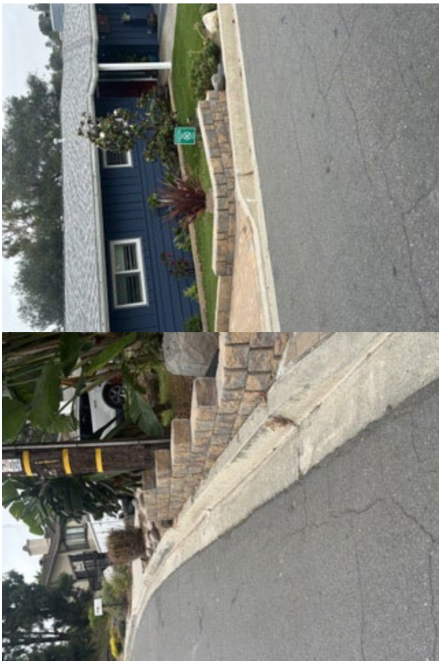
Water catch basin...you can see where the burn was dug through.
