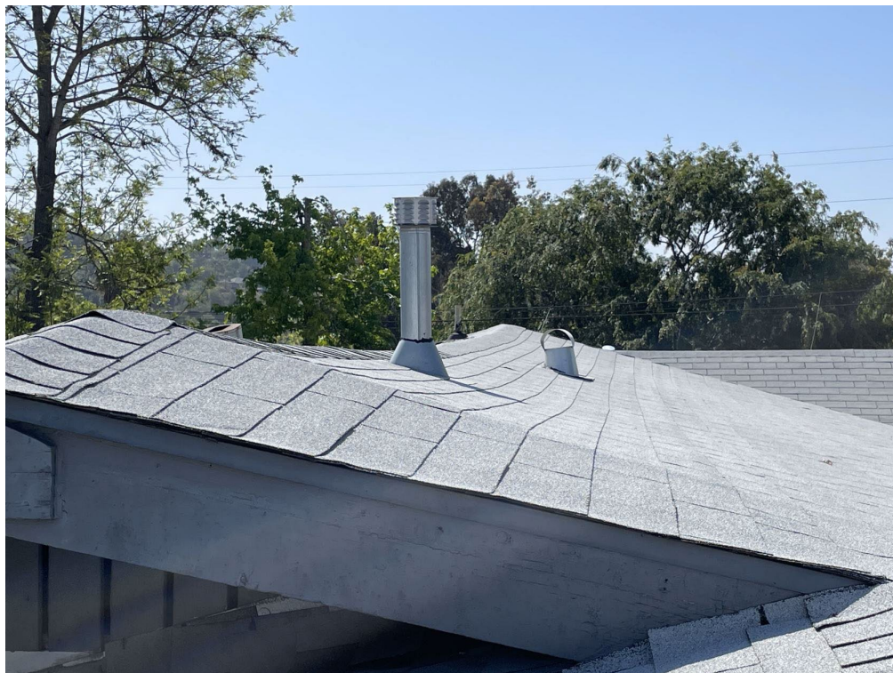
Roof Damage – Front of property
