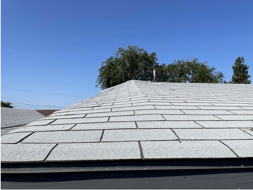
Roof Damage – Rear of Property
