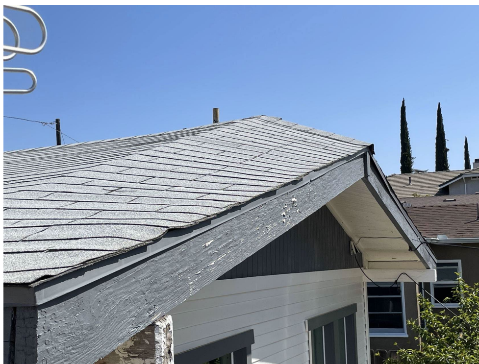
Roof Damage – Rear of Property
