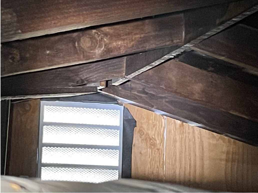
Roof Damage - Interior
