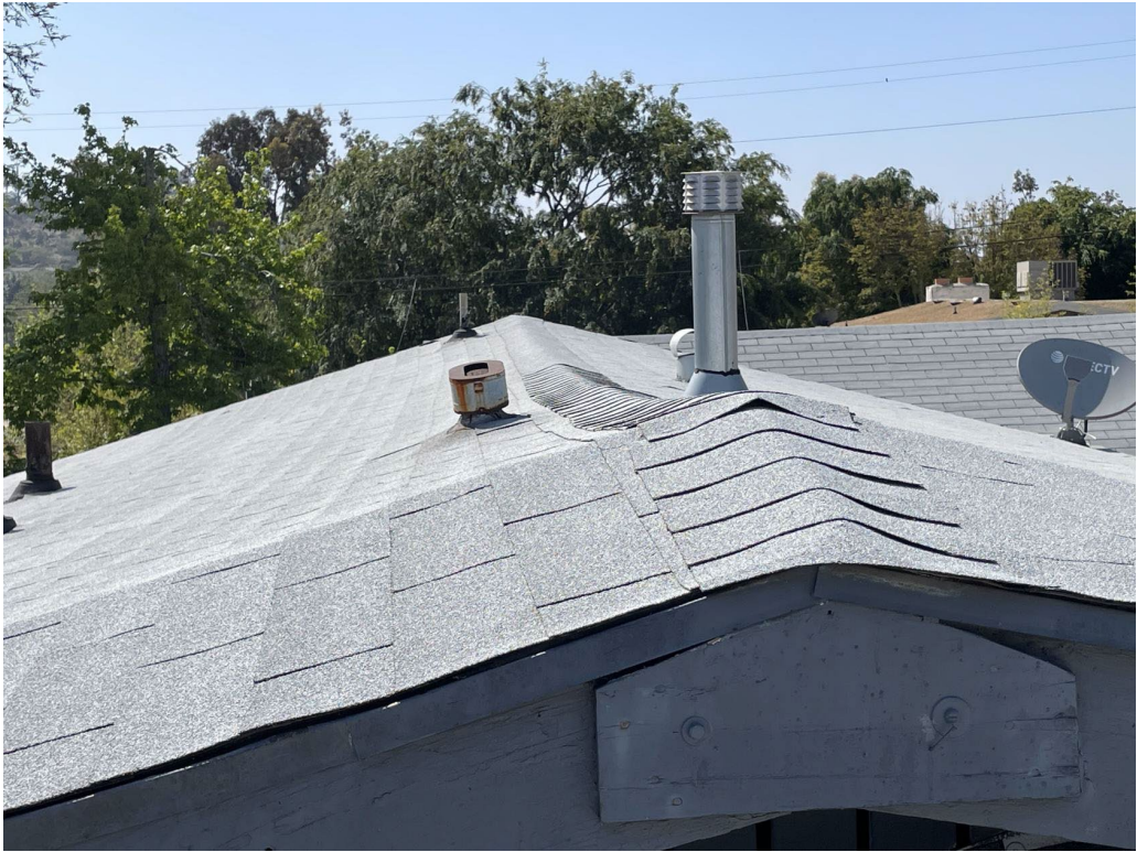
Roof Damage – Rear of structure
