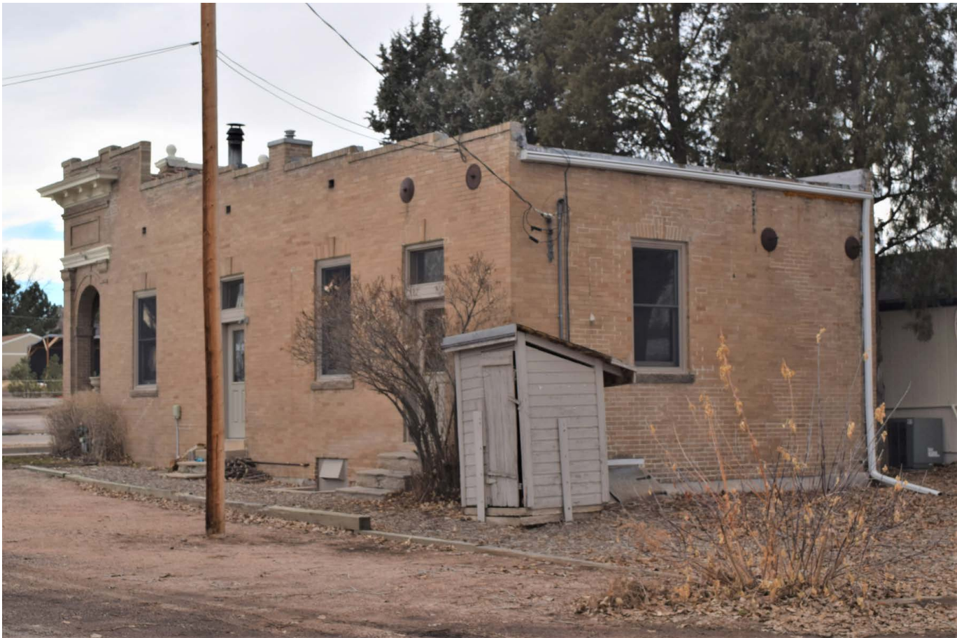
South and Rear elevations of 188 S. Main Street, stepped parapet and secondary doors visible, outhouse is presumed to be original Photo source: Town of Elizabeth
