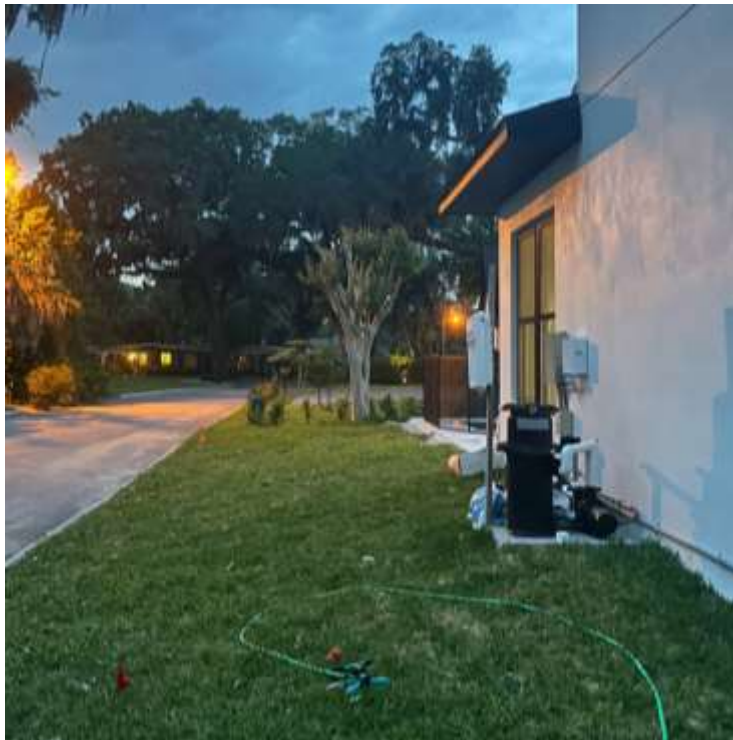
Exhibit 3 – Existing Pool Equipment (looking north from Oak Lynn/Haverill Road on the left)
