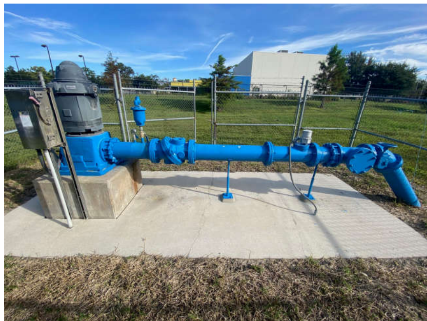
Photo 4-1: Wellhead Discharge Assembly
