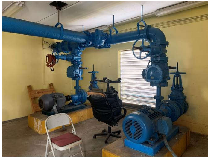
Photo 4-4: High Service Pumping
