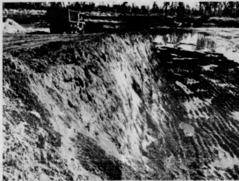
Digging presents a contrast in tone and texture. Truck moves down ramp (upper left) to be loaded.
