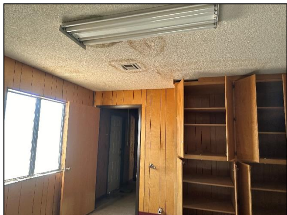
Water Leak Stains (Building C)
