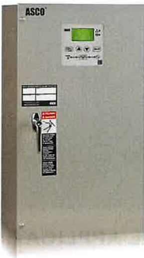
Fig. 1: ASCO Power Transfer Switch rated 200 Amps
