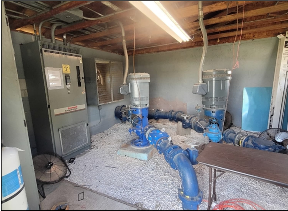
Figure C-3. Riner WTP High Service Pump Station
