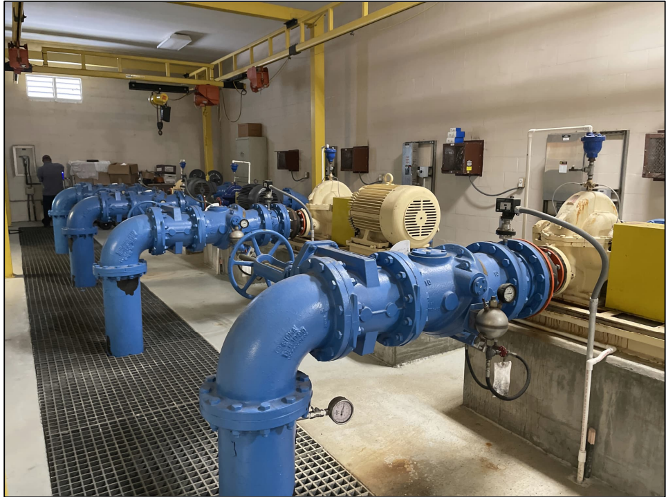
Figure C-1. Hickory Walk WTP High Service Pump Station
