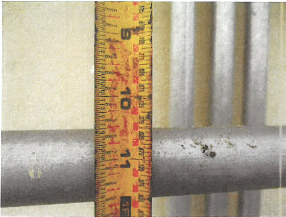
Ladder Rungs (note lack of anti-skid surface)
