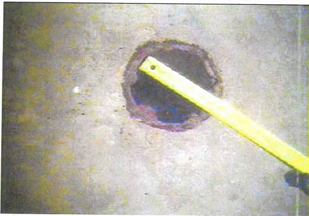
Floor Drain (note rust nodules at perimeter)
