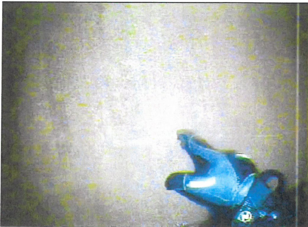
Minor Cracking on Upper Wall
