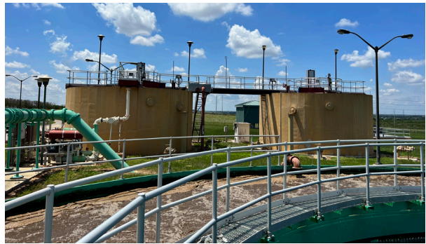
DIGESTERS AT WWTF
