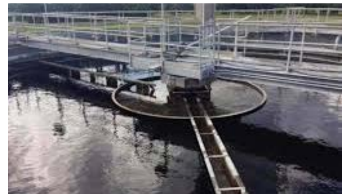
Figure 9. South Regional Water Reclamation Plant
