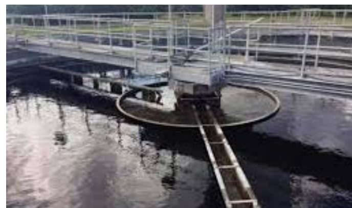
Figure 9. South Regional Water Reclamation Plant
