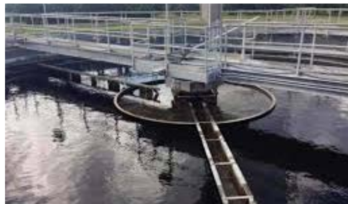
Figure 9. South Regional Water Reclamation Plant
