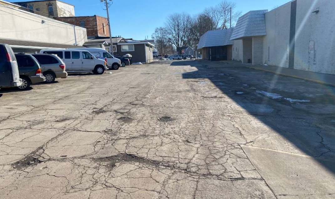
Photo 4: View of asphalt problems in north parking lot.
