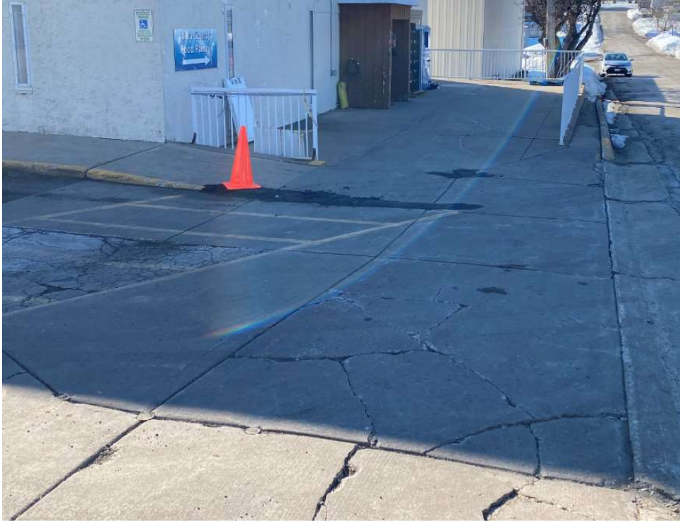
Photo 1: Concrete area west of SWCAP building. Asphalt patching was placed in an attempt to correct drainage issues.
