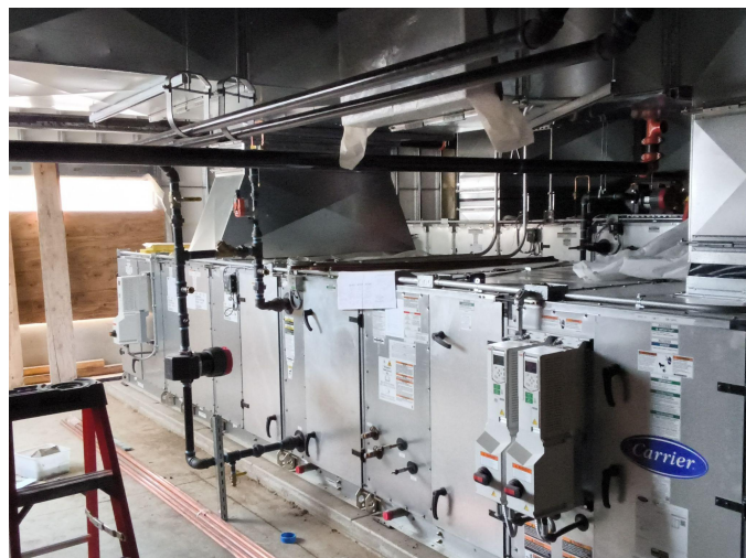
Air handling units
