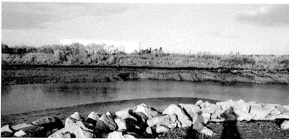
Figure 9: Looking west from harbor at the erosion adjacent to the fuel tanks
