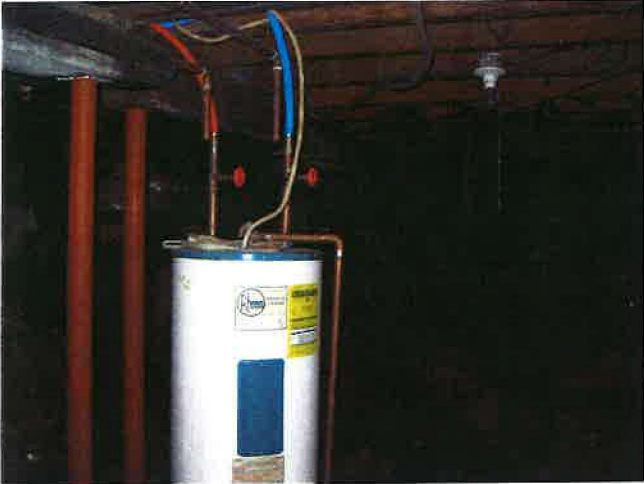
Water Heater in crawl space
