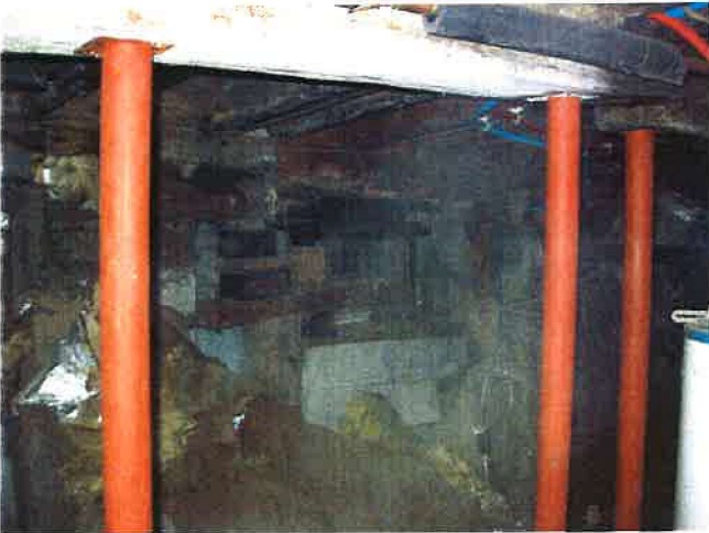
See the stacked up block and timbers for the exterior foundation wall in the distance, note the mold again
