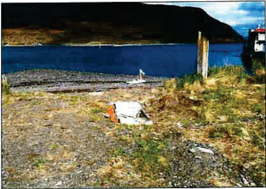
Photograph 2. Typical Beach Manhole
