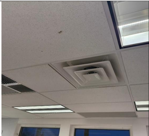
Forced Air heating
