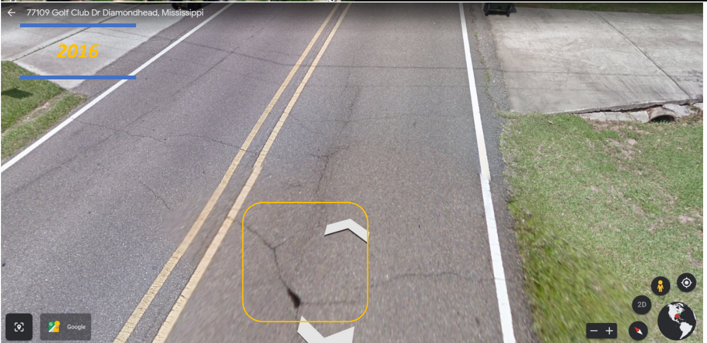
Same cracking visible in both 2016 and current imagery.
