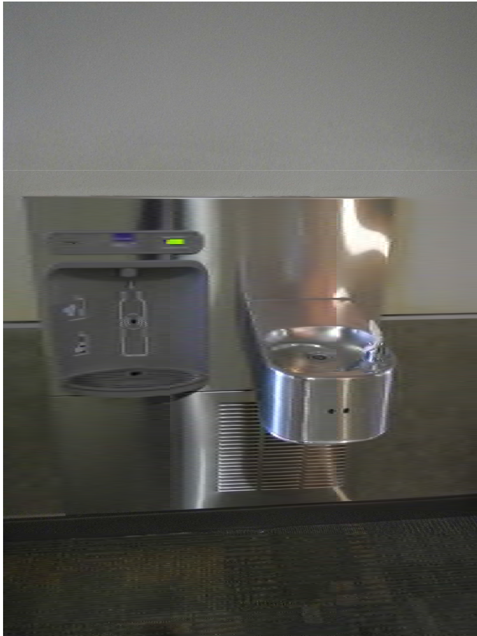
Figure 17 : Water bottle filling station and drinking fountain in holdroom
