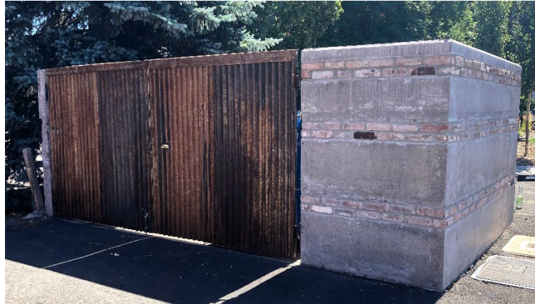
Figure 8: This trash enclosure is constructed of nonflammable materials (i.e., masonry brick wall, corrugated metal panel gates), 310 E Cascade Avenue.
