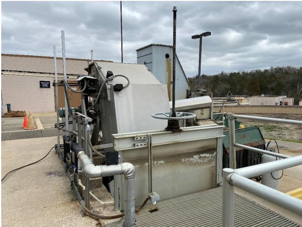
Mechanical Screen and Inlet Gate
