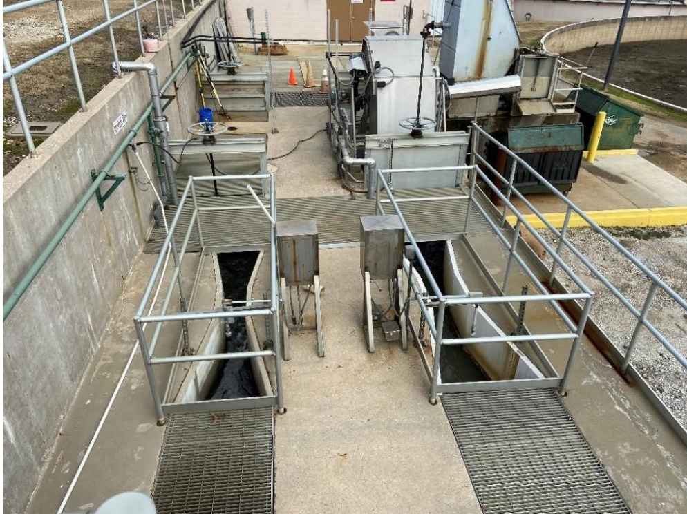
Duck Creek (Left) and Combined Paw Paw and Iron Ore (Right) Parshall Flumes
