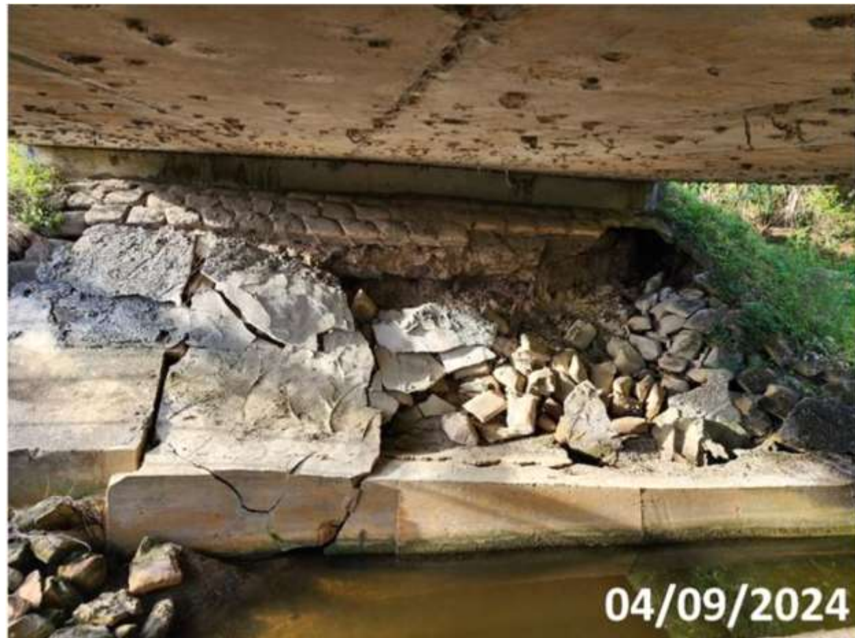
Photo 6: Element 8396: Abutment 1 slope failure (80% bags scoured out).
