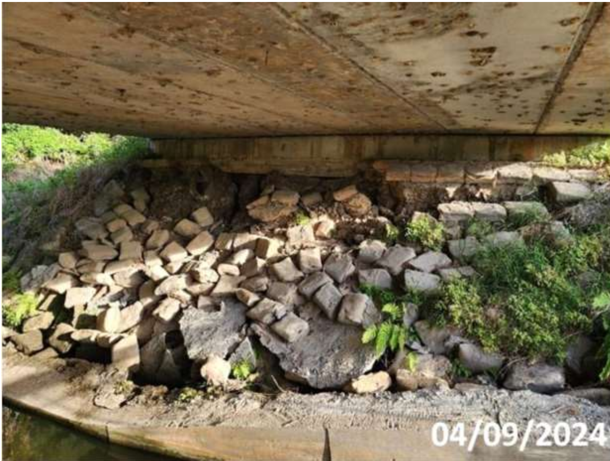
Photo 7: Element 8396: Abutment 2 slope failure (95% bags scoured out).
