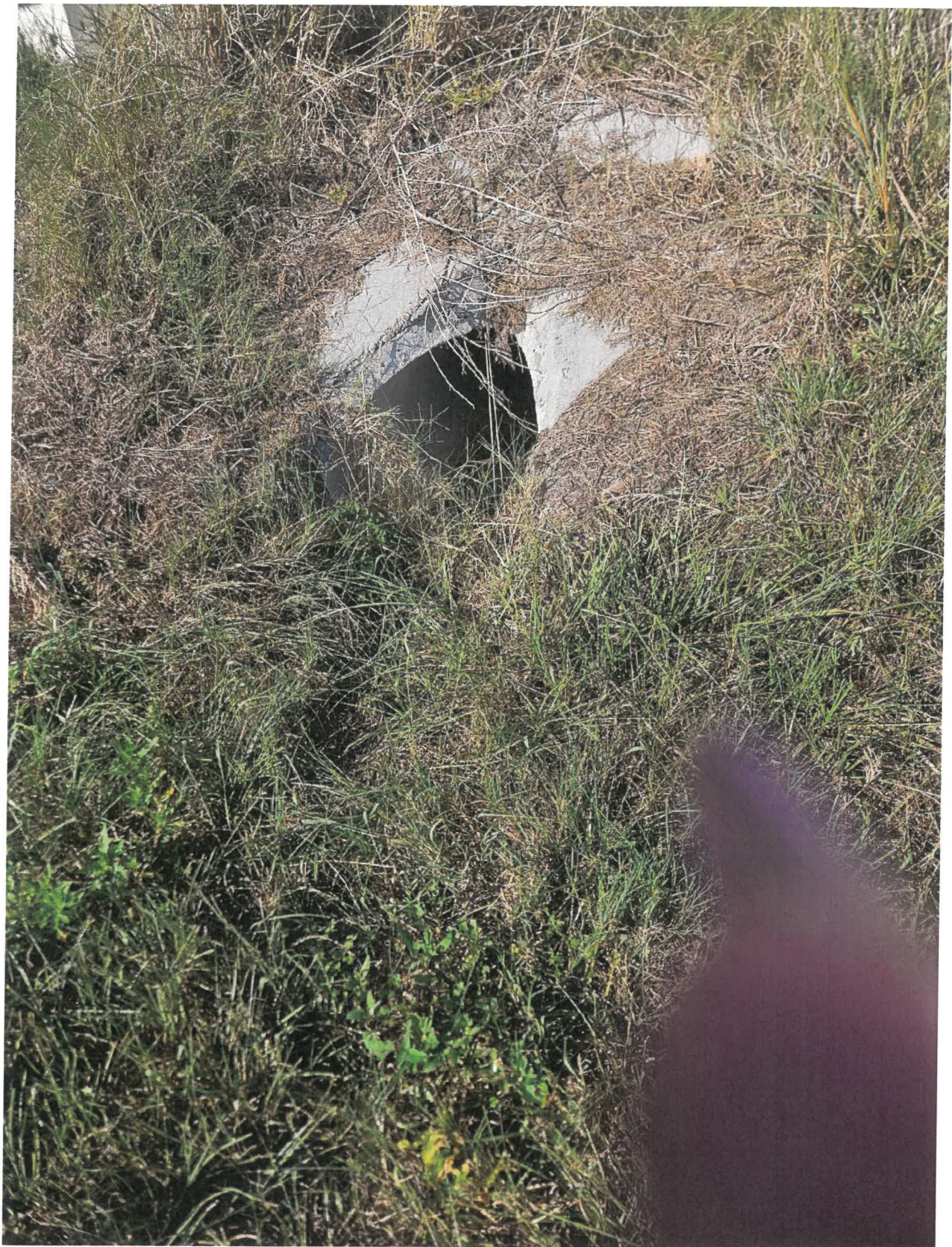
Culvert on pond side over grown and higher than on the ditch side. Dry as a bone.
