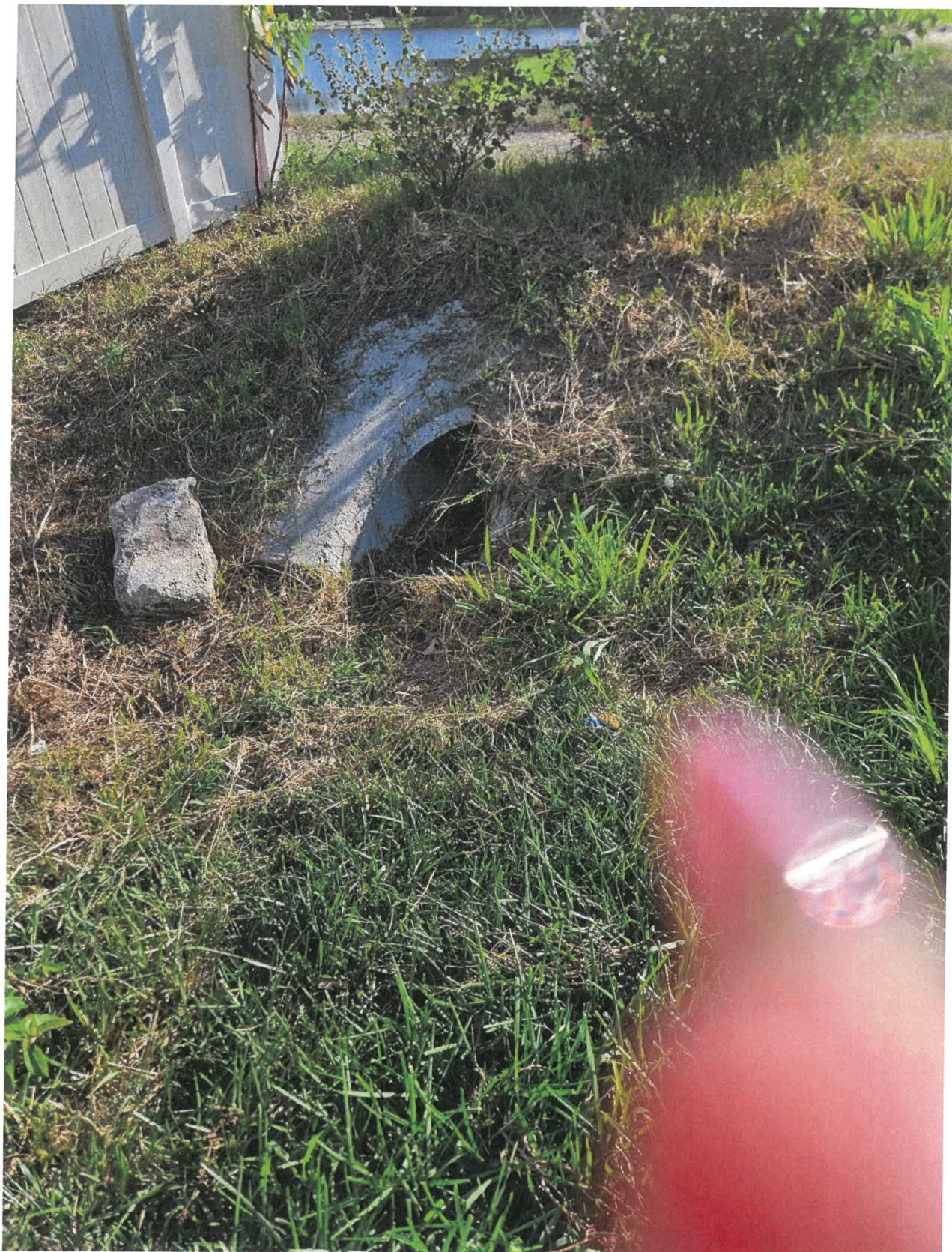
Overgrown Culvert on ditch side. Owners here have been trying to clean the area themselves.
