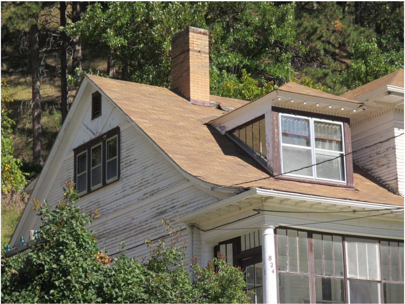
Displaced shingles and peeling paint observed 09-24-15
