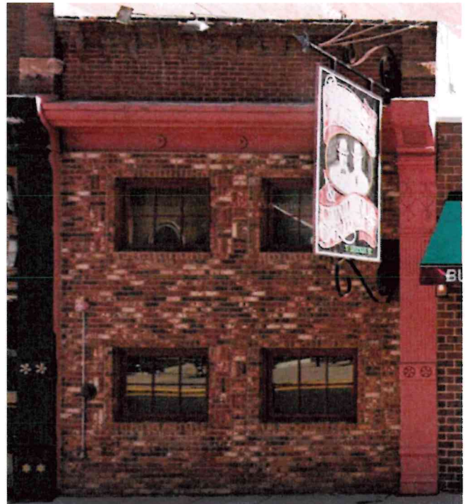
CURRENT STOREFRONT – Replace with new wood storefront like original. Storefront can be designed to accommodate a new entrance in the future. Anticipate an awning like The Landmark.
