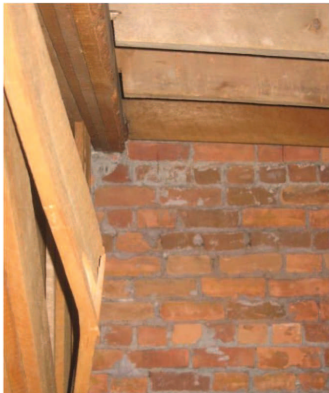
Photo No. 32: Girder truss to the east of subject girder truss. Breakage of the first panel diagonal at the north end.
