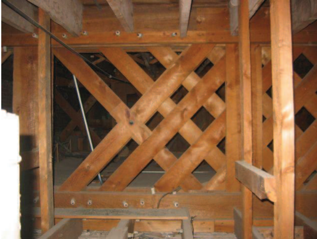
Photo No. 29: View of girder panel at south end of girder truss.
