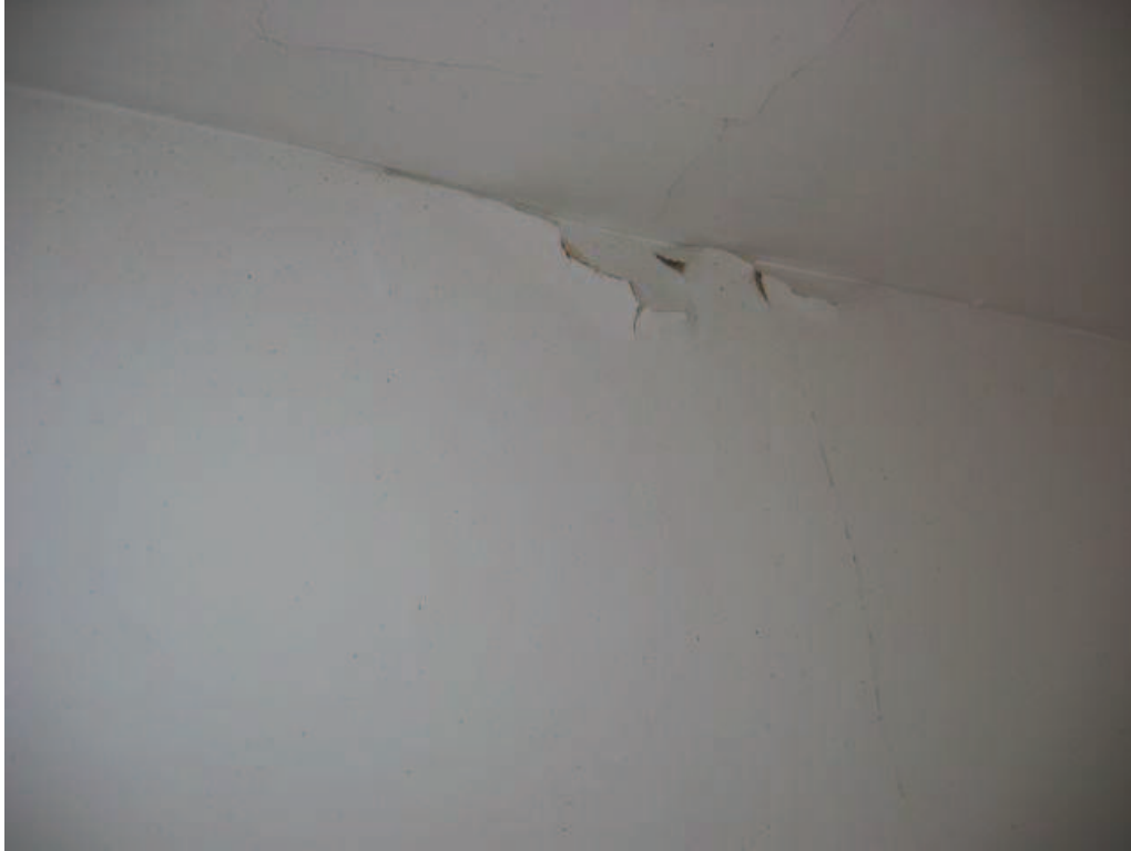
Photo No. 7: Crackage at ceiling in hallway at south end of girder truss.
