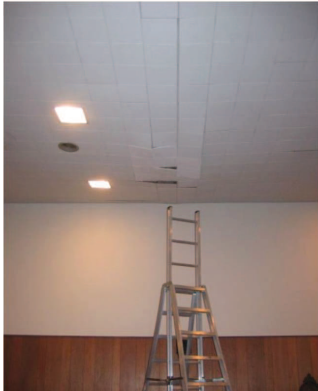
Photo No. 1: Displaced ceiling tile in auditorium at north end of girder truss.
