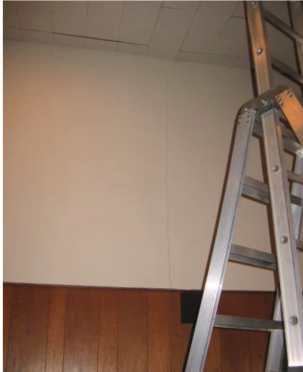
Photo No. 3: Plaster crackage at north wall of auditorium under girder truss bearing.
