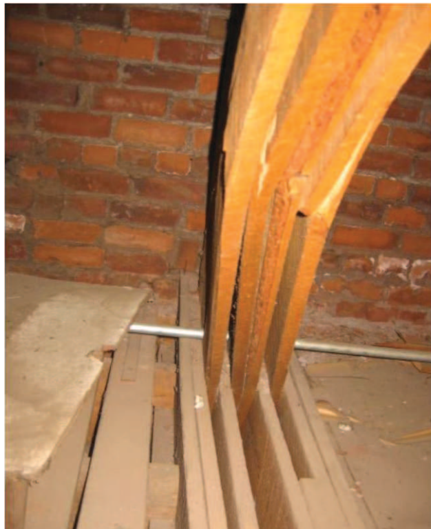
Photo No. 20: View of diagonal breakage at south end of girder truss.
