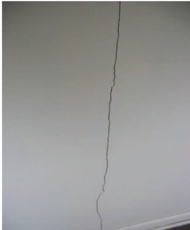
Photo No. 8: Crackage in plaster at hallway on south side of building under the girder truss bearing.
