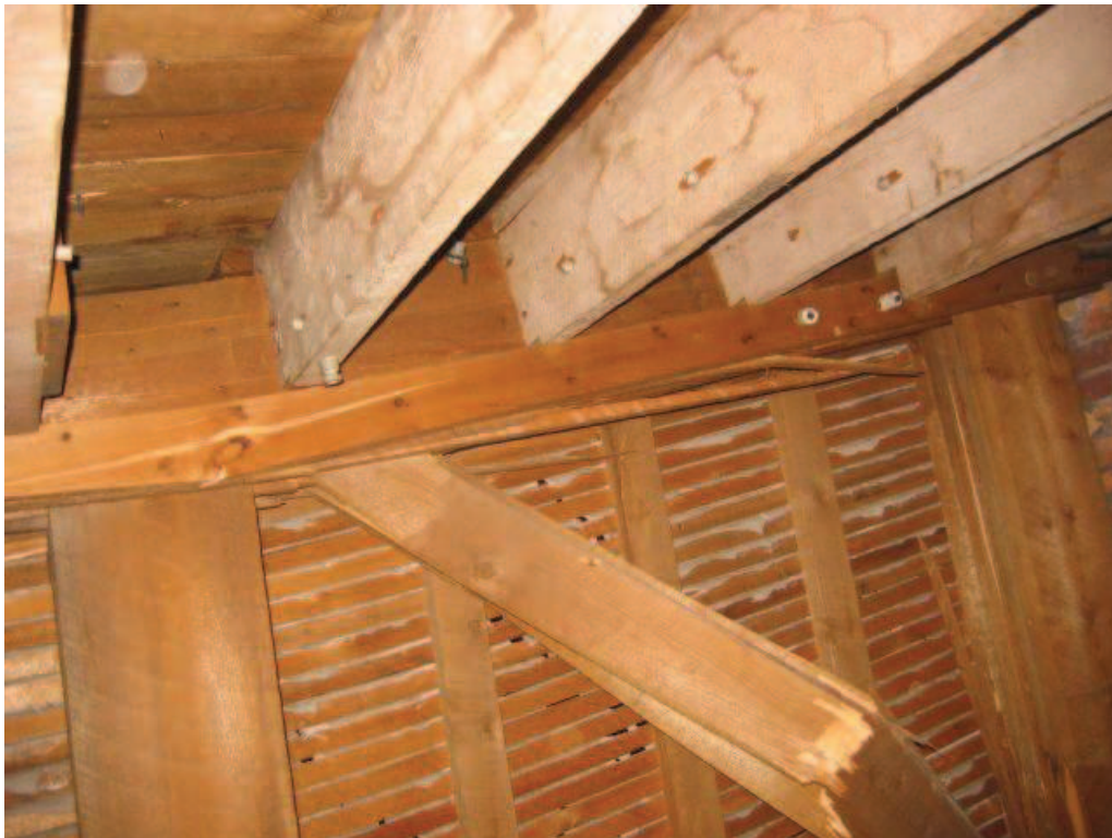
Photo No. 10: Breakage of the top chord boards at the north end of the girder truss.
