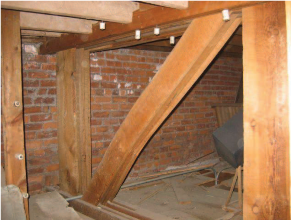
Photo No. 15: Breakage of the diagonal at south end of girder truss.
