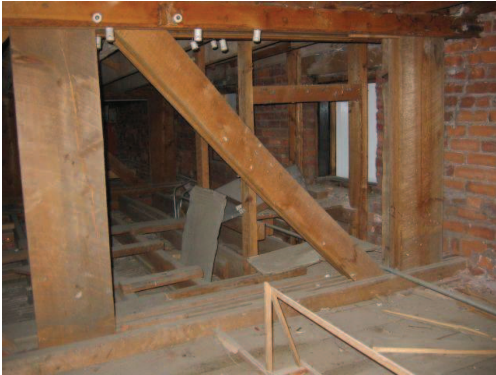
Photo No. 17: Breakage of the vertical chord member at south end of girder truss.
