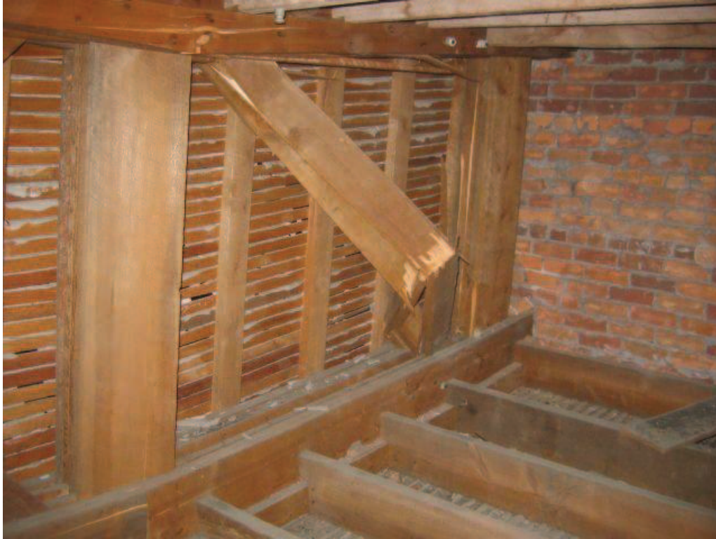
Photo No. 9: Overall view of broken girder truss members at north end of girder truss.
