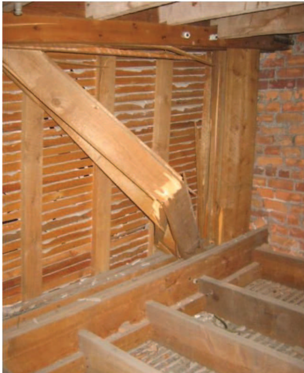
Photo No. 12: Breakage of diagonal chord member at north end of girder truss.
