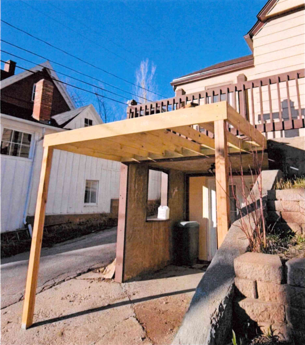
Addition to existing concrete deck. 6x9 Trex and cedar handrail with black baluster.
