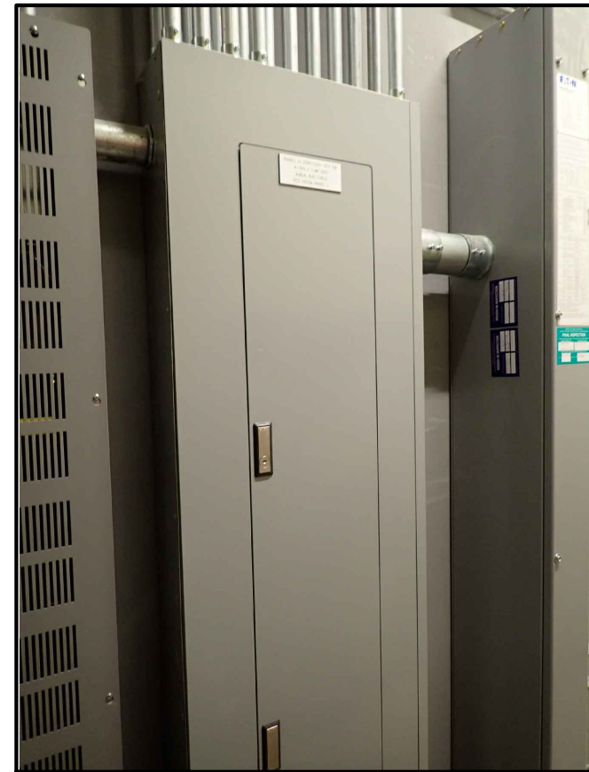
3 POWER PANEL PHOTO
