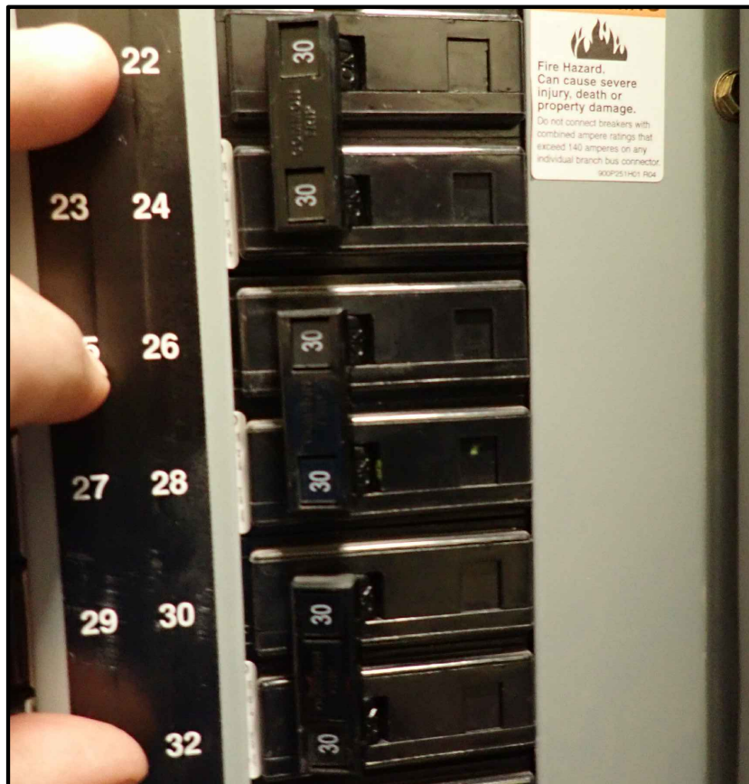
4 ELECTRICAL BREAKERS PHOTO
