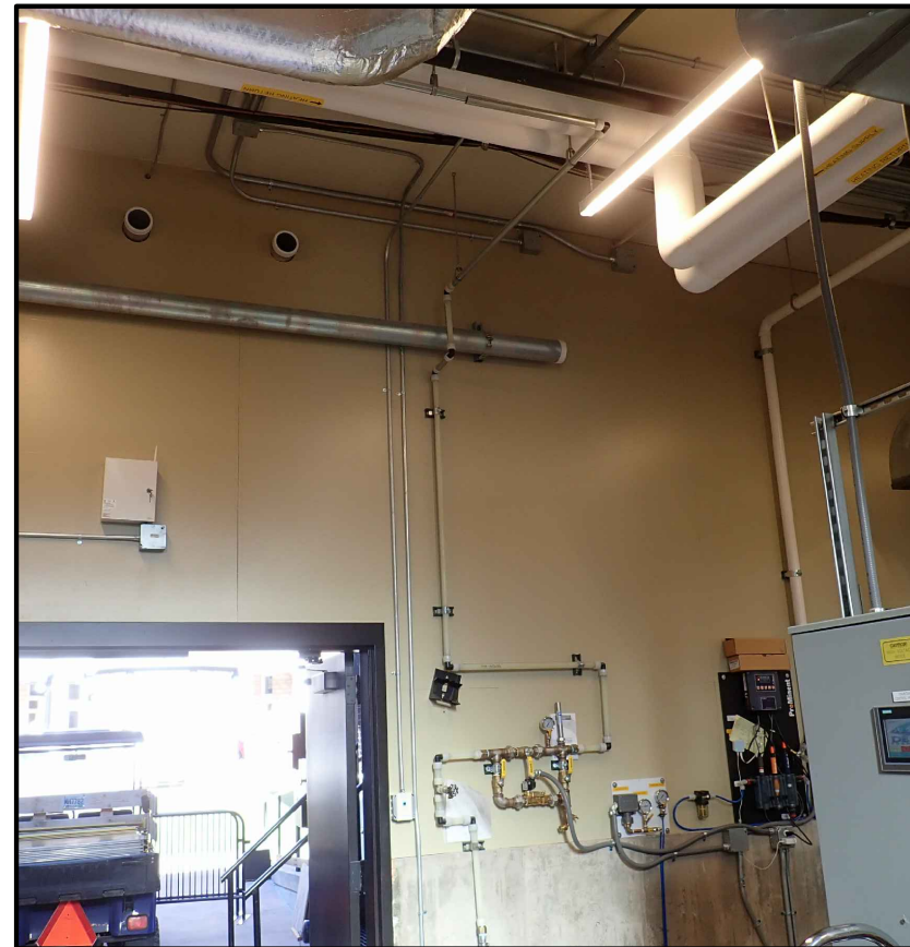
5 EQUIPMENT MOUNTING SPACE PHOTO
