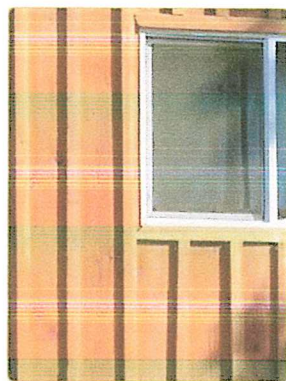
EXTERIOR SIDING : DOUGLAS FIR: ROUGH CUT Douglas Fir Board and batton detail of exterior siding installation.
