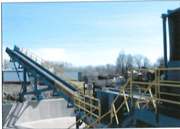
Figure 2. Shredder system conveyor.
