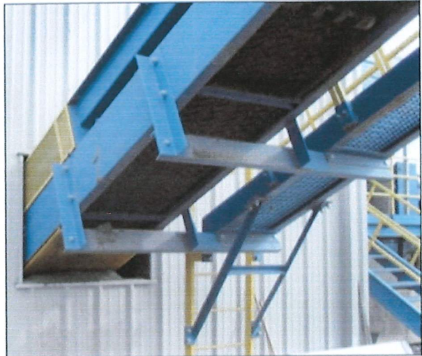
Figure 9. Shredder conveyor opening.
