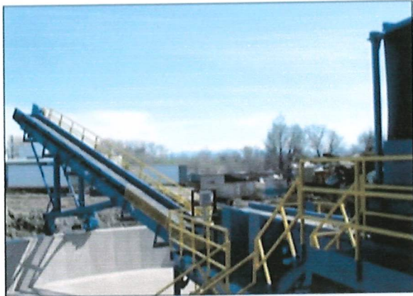
Figure 2. Shredder system conveyor.
