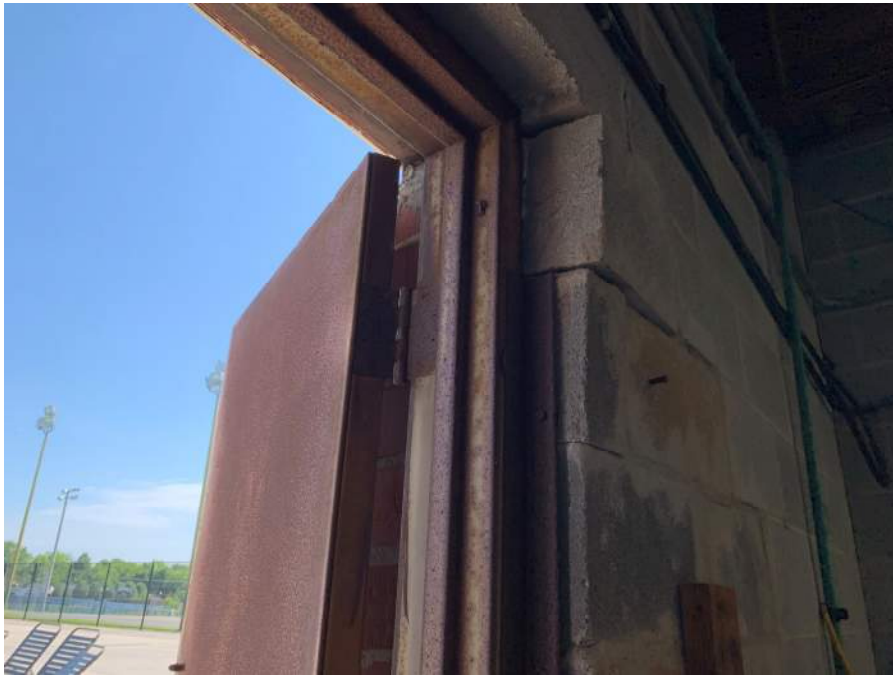
Photograph H: Building A Rusted Door Frame
