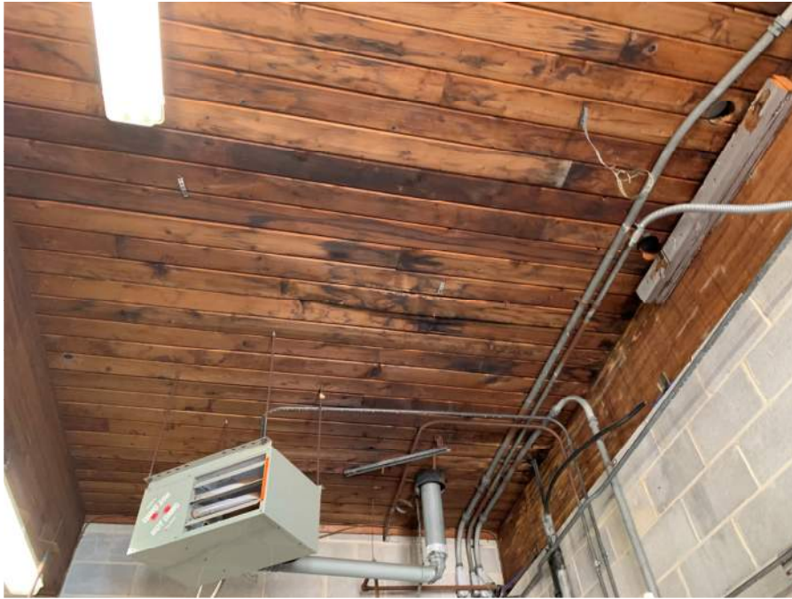
Photograph G: Significant Deflection on Building A Timber Decking Over Pool Mechanical Room (Looking South)
