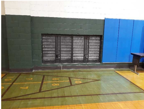
Gymnasium Ventilation Intake Louvers
