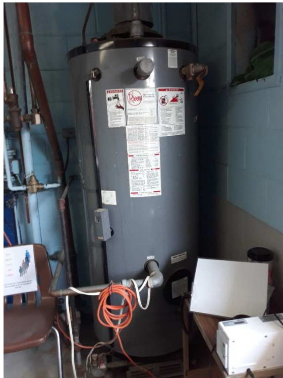
Pool Water Heater for Showers
