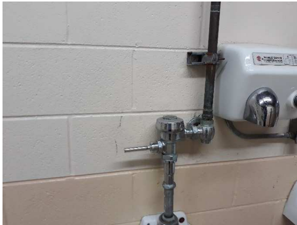
Locker Room Piping indicating corrosion
