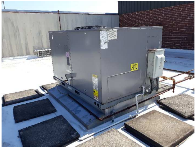
Rooftop Unit for Original Building
