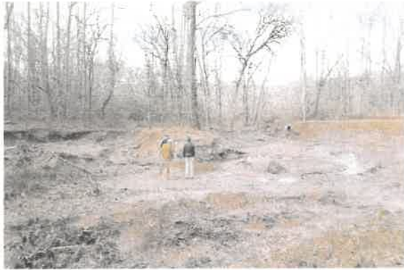
Stream was excavated for an unpermitted pond
