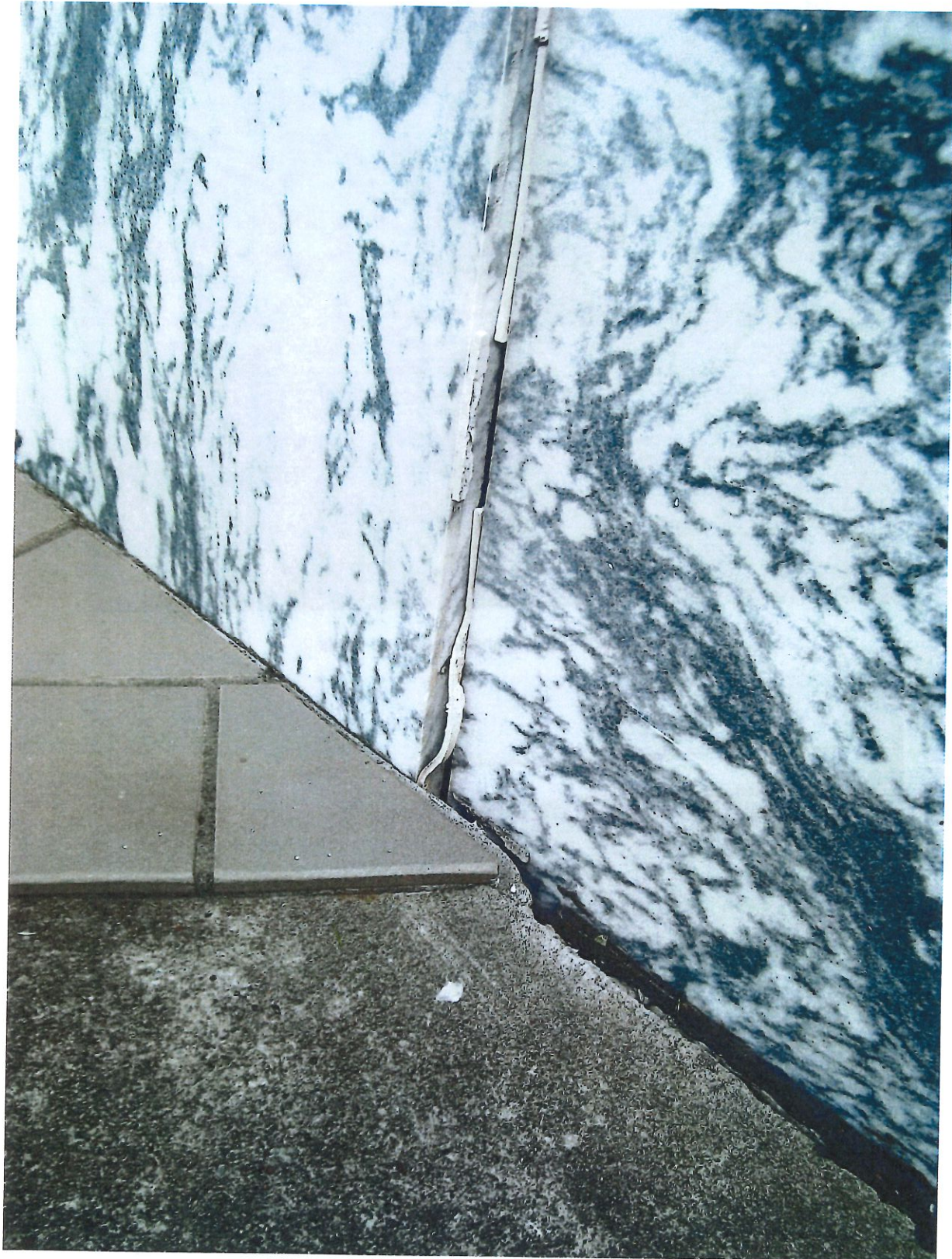
Repair sag, re-caulk 2
