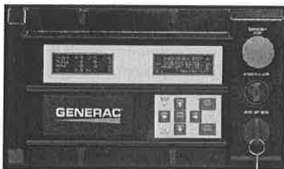
Digital H Control Panel—Dual 4x20 Display
