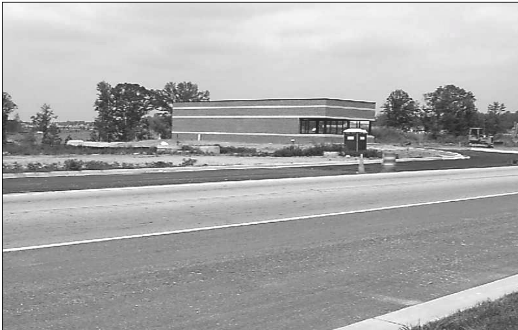
Waffle House under construction on the south side of SR 53 east of Georgia 400
