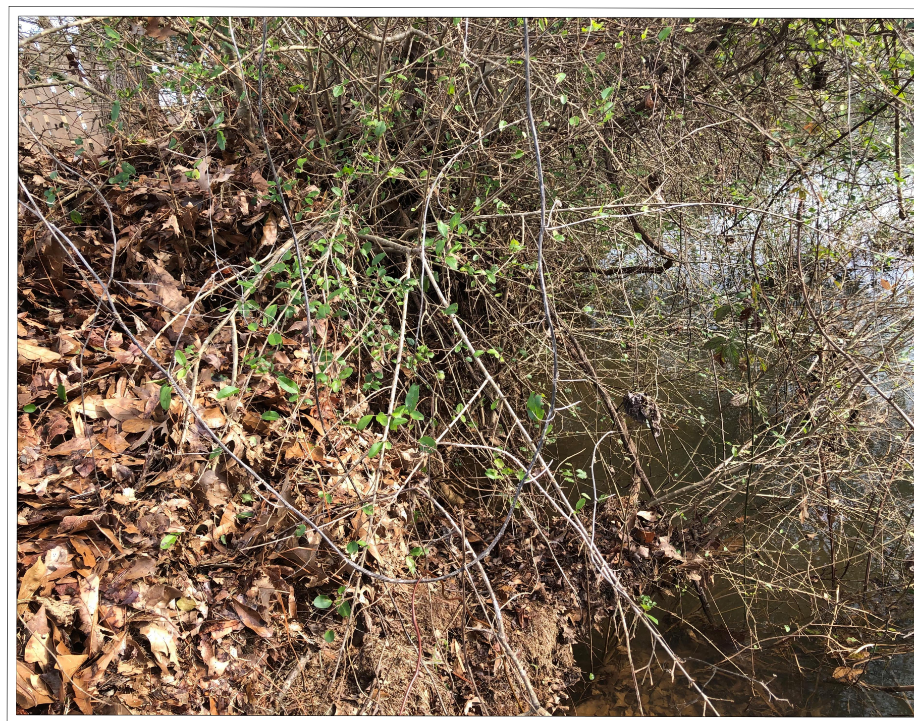
PICTURE "3" RIVER BANK ERODING
