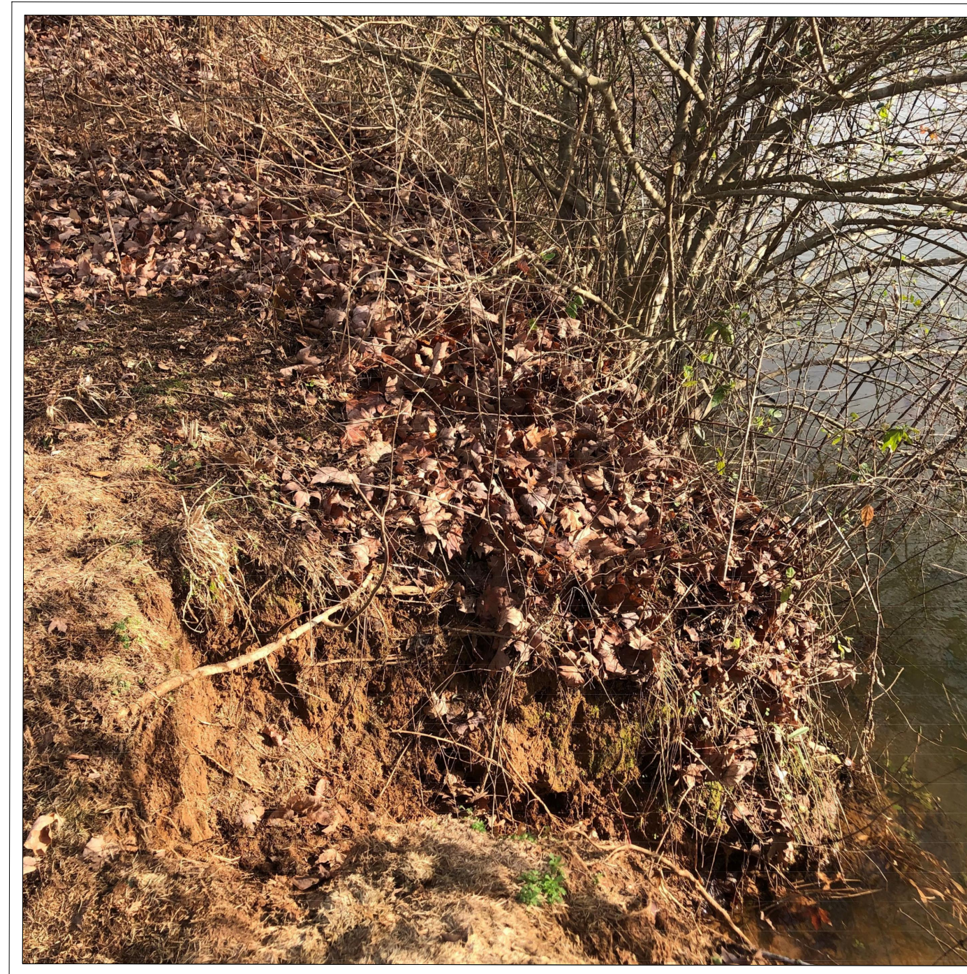
PICTURE "1" RIVER BANK ERODING
