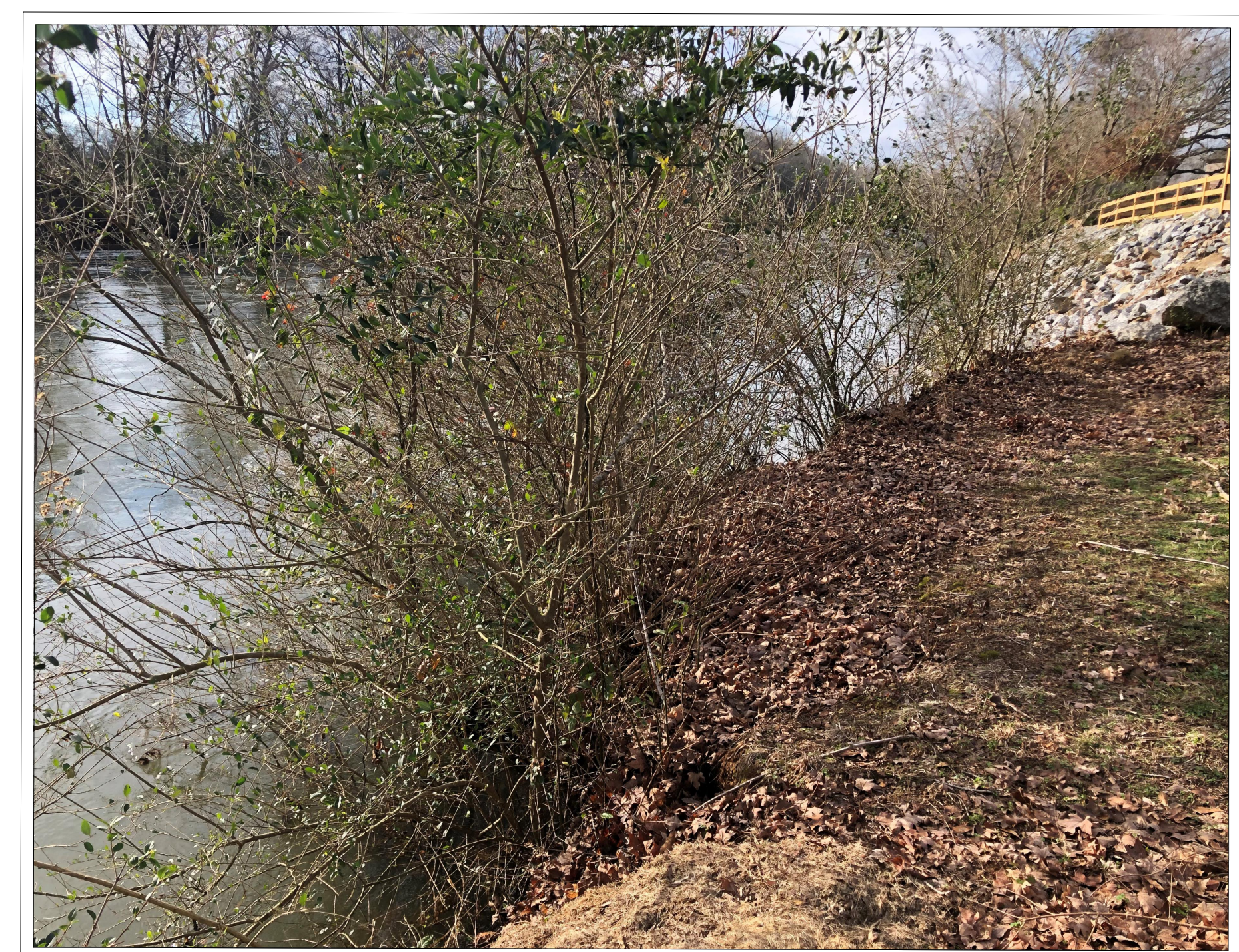
PICTURE "4" RIVER BANK ERODING
