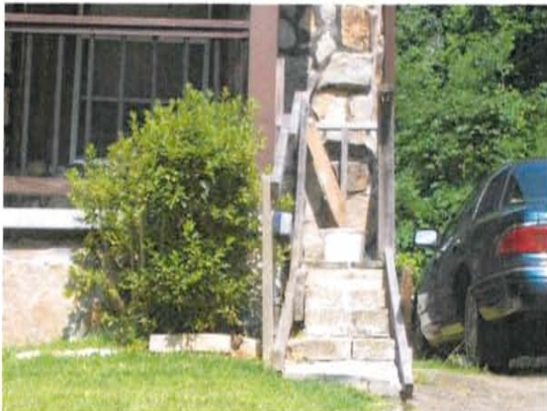
These front steps need to be replaced.
