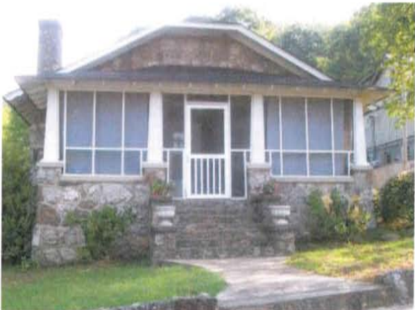
This porch has been enclosed which takes away from the historic character of the house.
