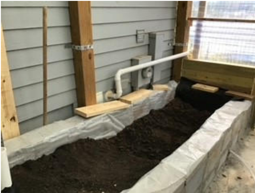
Electric meter is inside the greenhouse.
