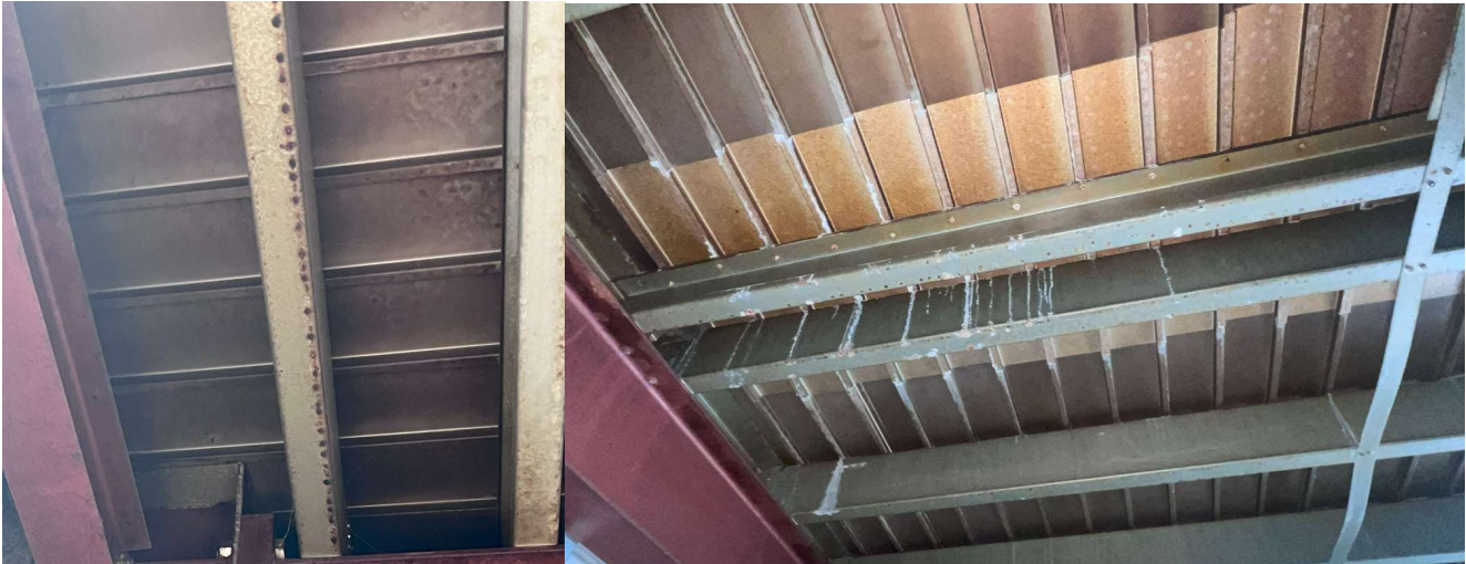
Corrosion/Rusting of Light Gage Joists Below 2 nd Floor Concrete Deck
