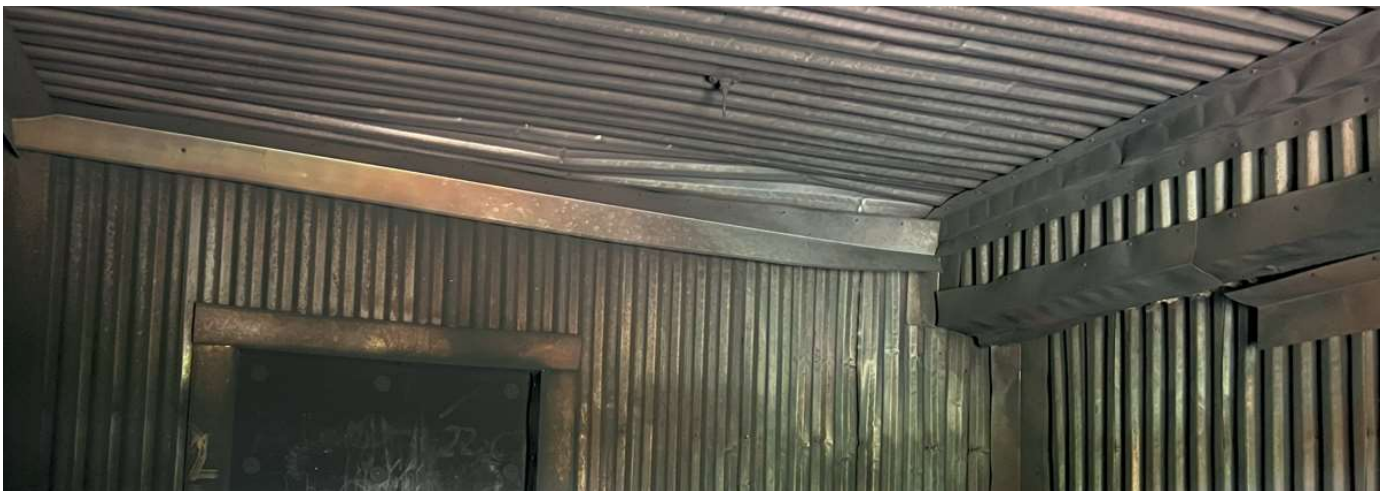
Burn Room #2 Warped Ceiling Panels & Trim / Northwest Wall Panel Heavily Warped & Discolored
