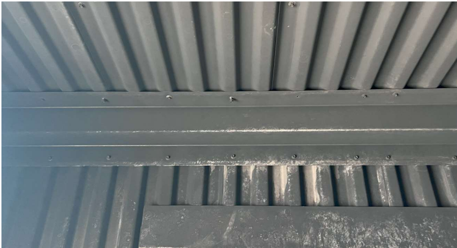
Backed out & Missing Ceiling Trim Screws
