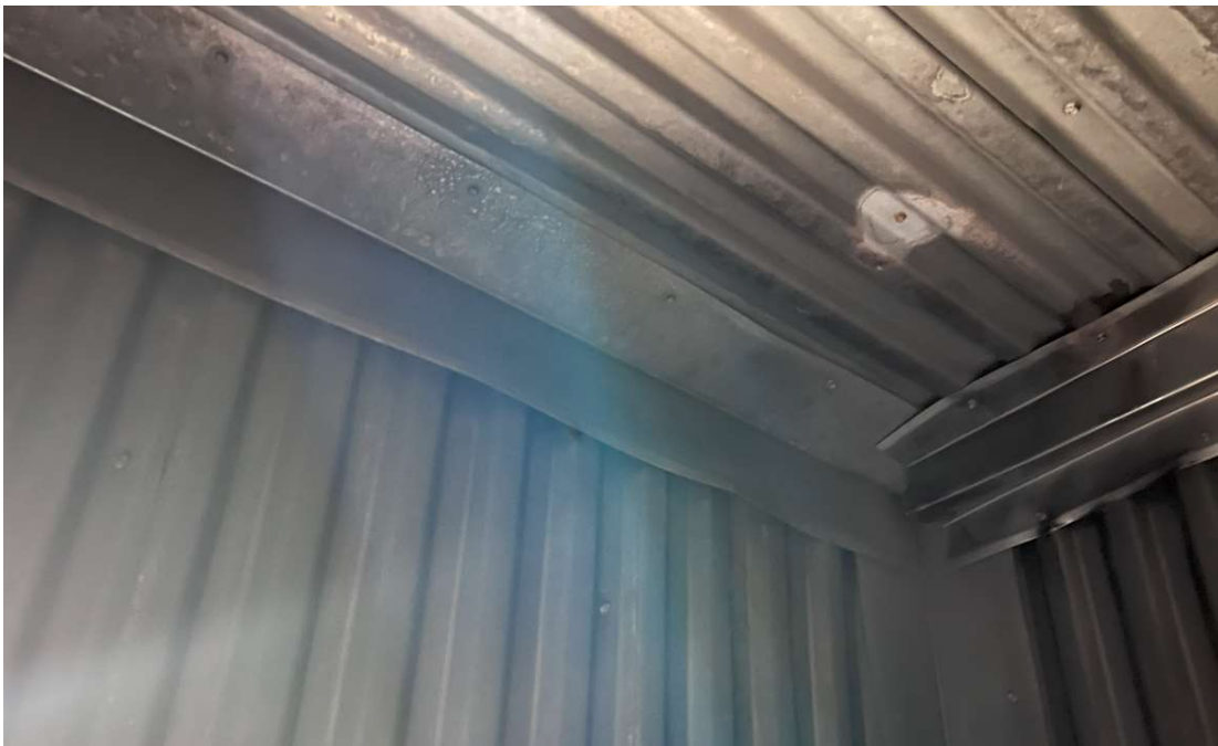
Burn Room #3 Corner Trim Missing Screws
