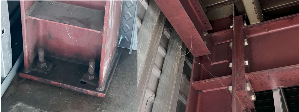
First Floor Columns & Baseplates Exhibiting Rusting/Paint De-lamination
