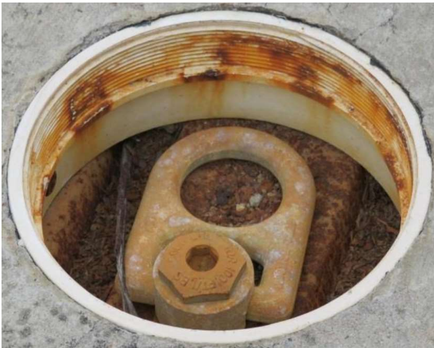
Rusted Rapelling Anchor
