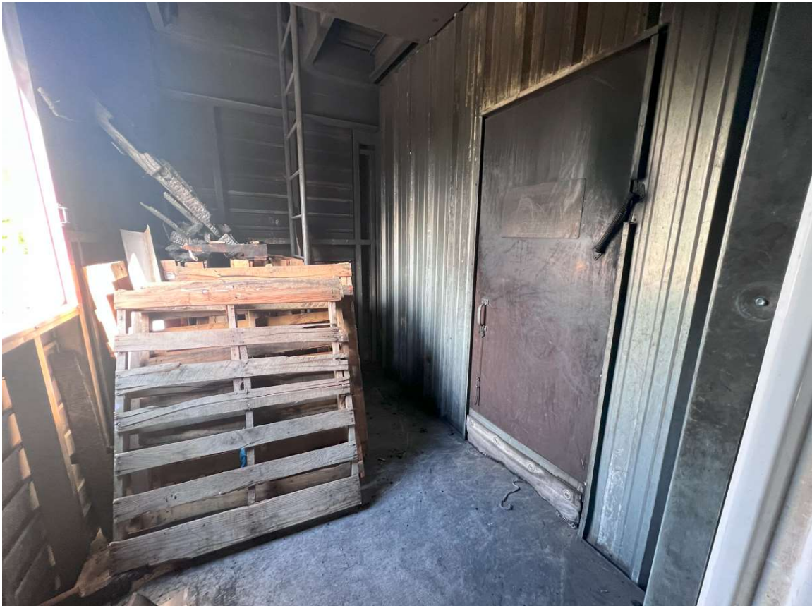
Fuel Source Stored Adjacent to 2 nd Floor Burn Room
