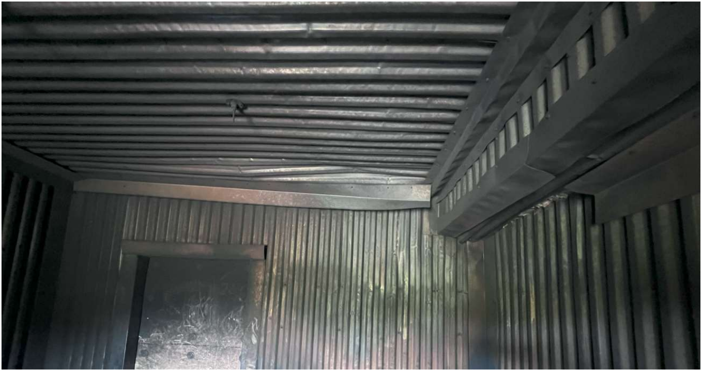
Burn Room #2 Warped Ceiling Panels & Trim
