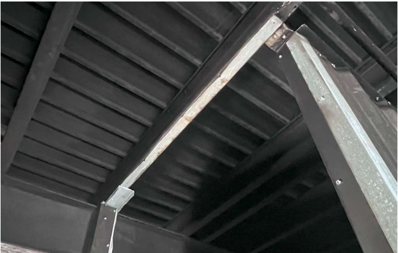
3 rd Floor Floor Joists & Deck (Soot Buildup & Rust)
