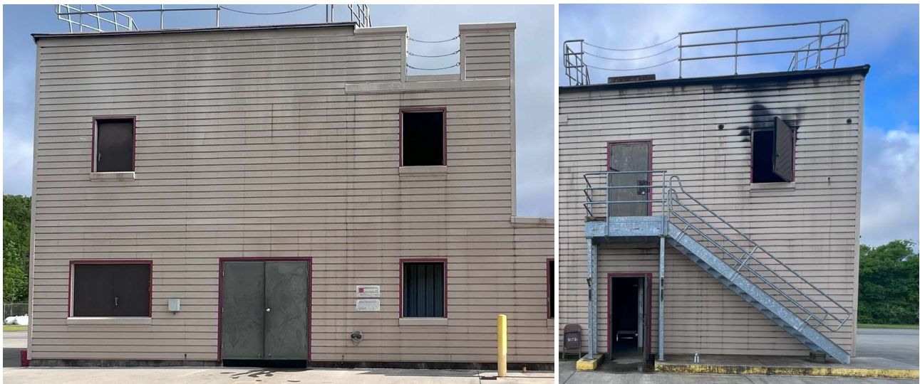
Rust Marks Along Screw Lines at Exterior Wall Panels/Soot Buildup Adjacent to 2 nd Floor Burn Room Door
